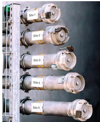
Silo Loading and Transfer lines
