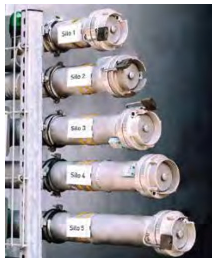
Silo Loading and Transfer lines
